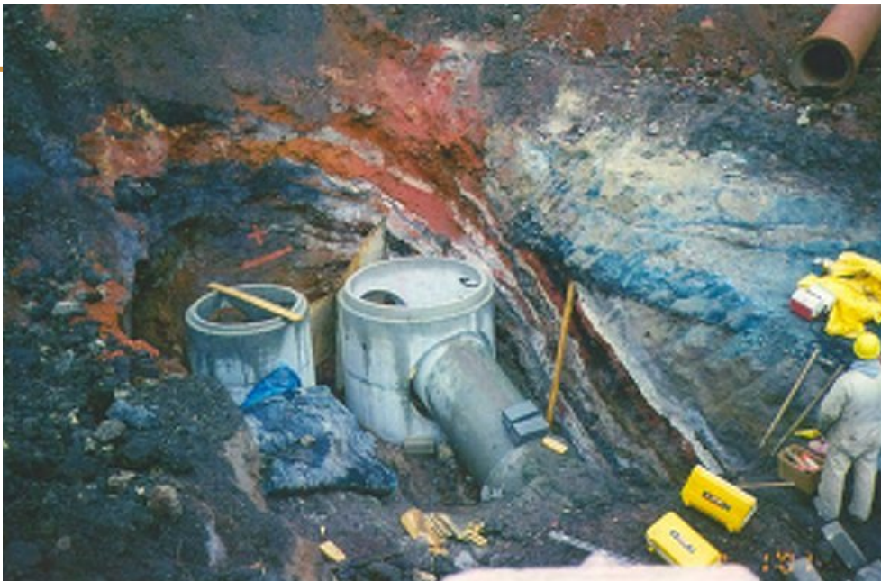
Utilities buried under the slag proved to be a challenging obstacle.
